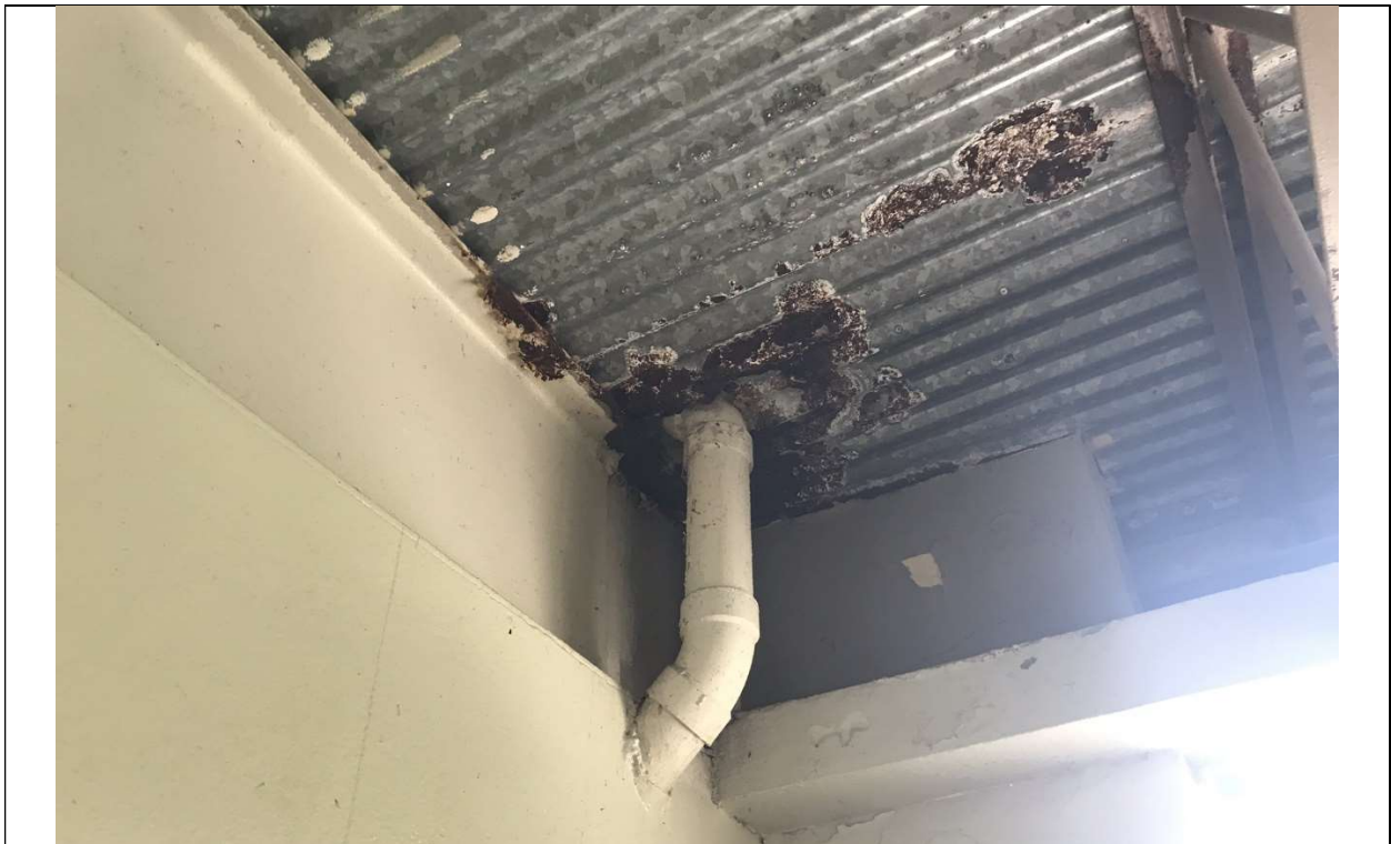
Picture 20 - Roof drains leak causing corrosion damages to steel components including metal deck on different levels
