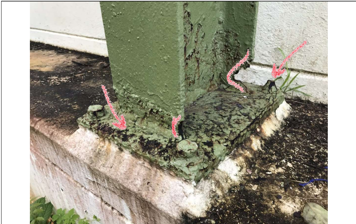
Picture 6 – Columns steel plate's anchor bolts and nuts significant loss of metal due to corrosion - Exterior perimeter columns
