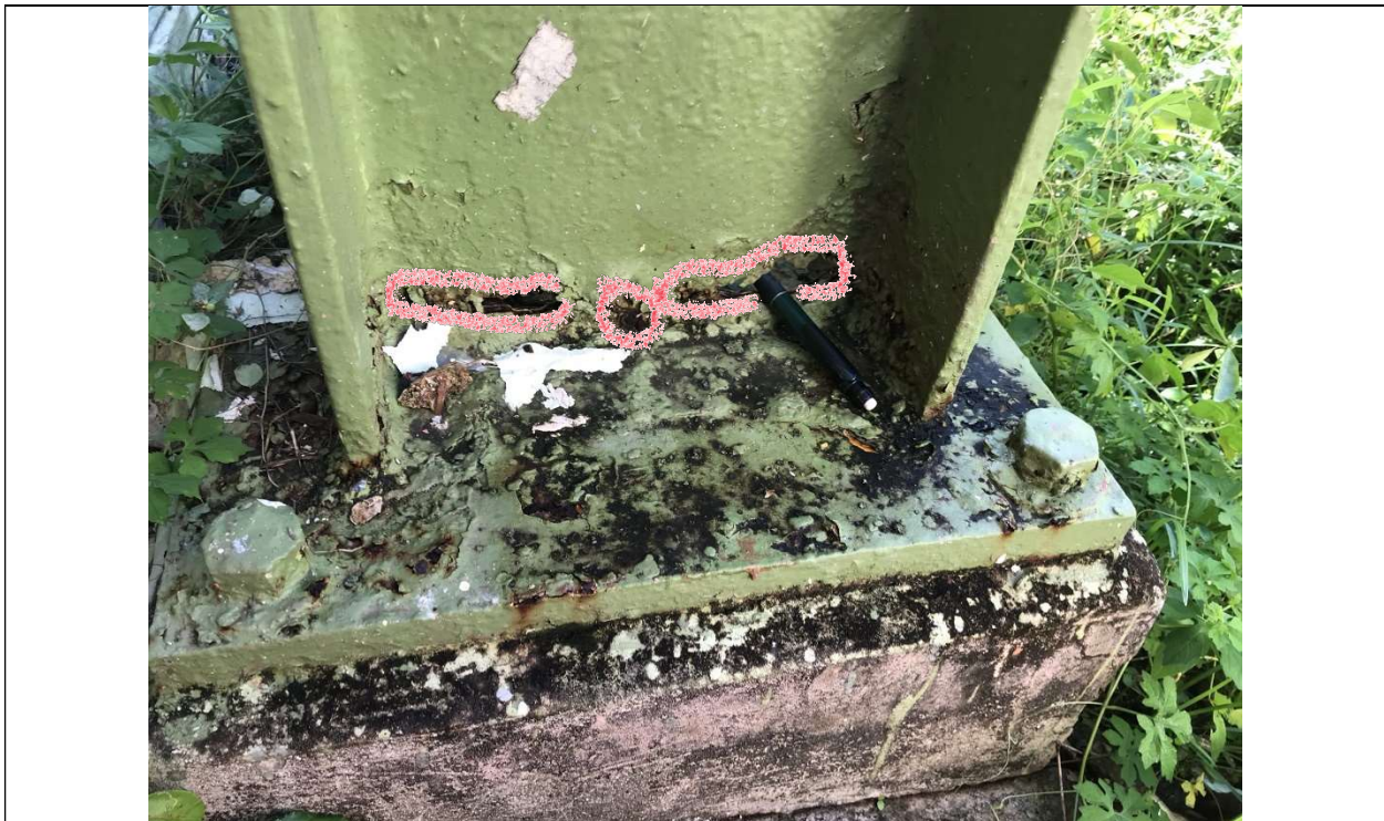
Picture 4 – Steel columns significant loss of metal at web and flanges within 12" of the plate due to extreme corrosion - Exterior perimeter columns
