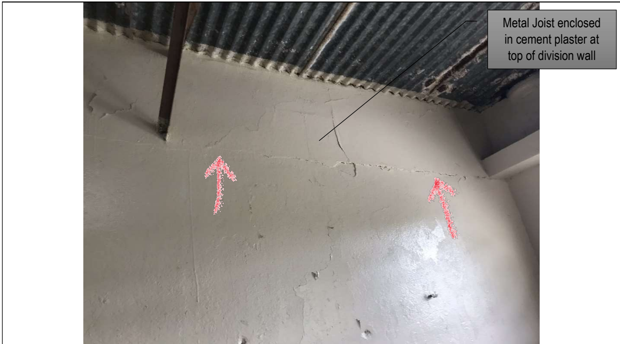
Picture 18 - Horizontal separation and/or cracks at masonry wall/ceiling intersection and other distances as measured down from the ceiling (Ex. At metal joist bottom level).
