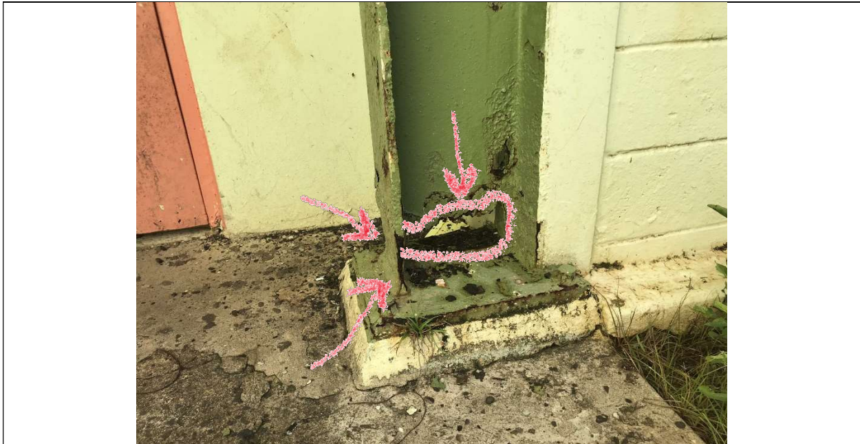
Picture 1 – Steel columns significant loss of metal at web and flanges within 12" of the plate due to extreme corrosion - Exterior perimeter columns
