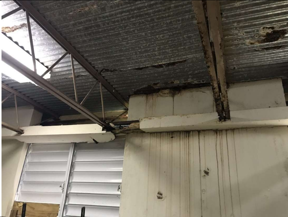
Picture 9 - Steel metal deck, joist and other related components badly corroded at a classroom on the 3rd floor of the bldg.'s West wing due to roof water leaks
