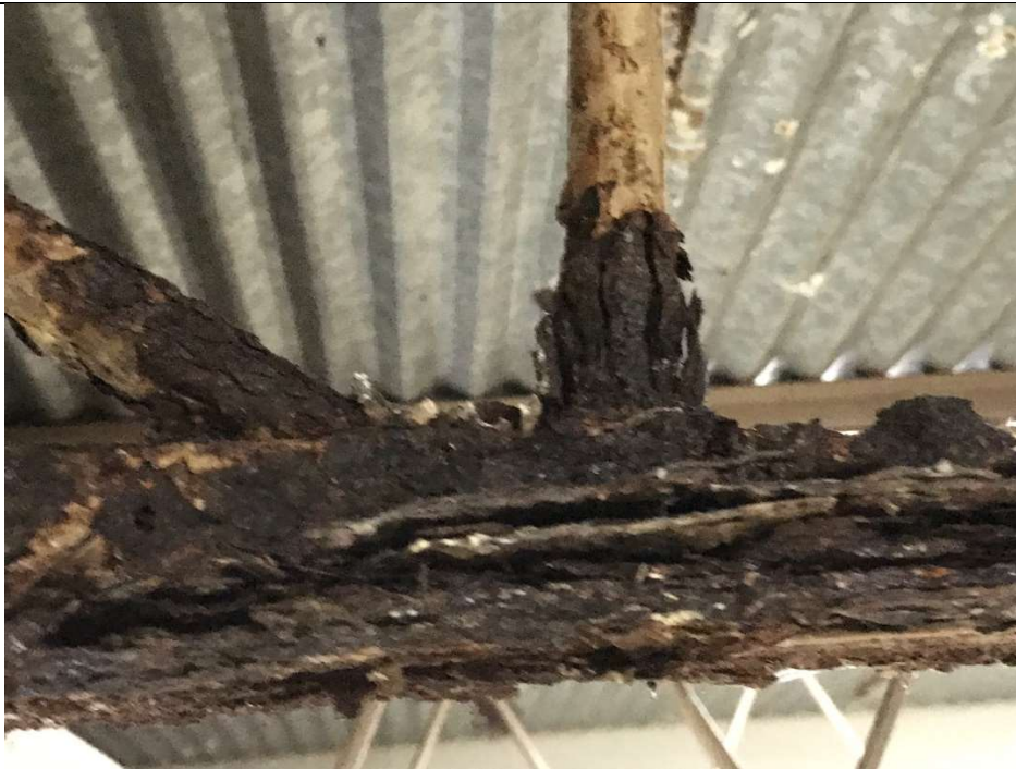
Picture 10 - Steel metal deck, joist and other related components badly corroded at a classroom on the 3rd floor of the bldg.'s West wing due to roof water leaks
