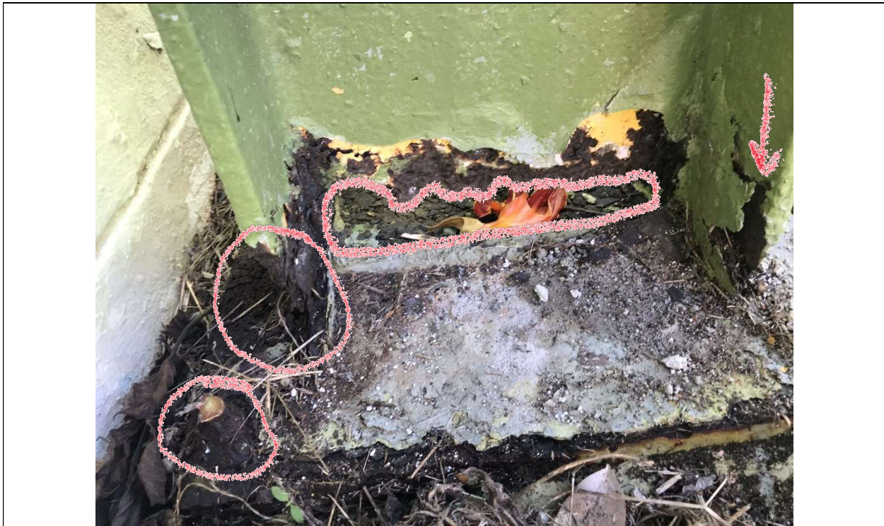
Picture 2 – Steel columns significant loss of metal at web and flanges within 12" of the plate due to extreme corrosion - Exterior perimeter columns
