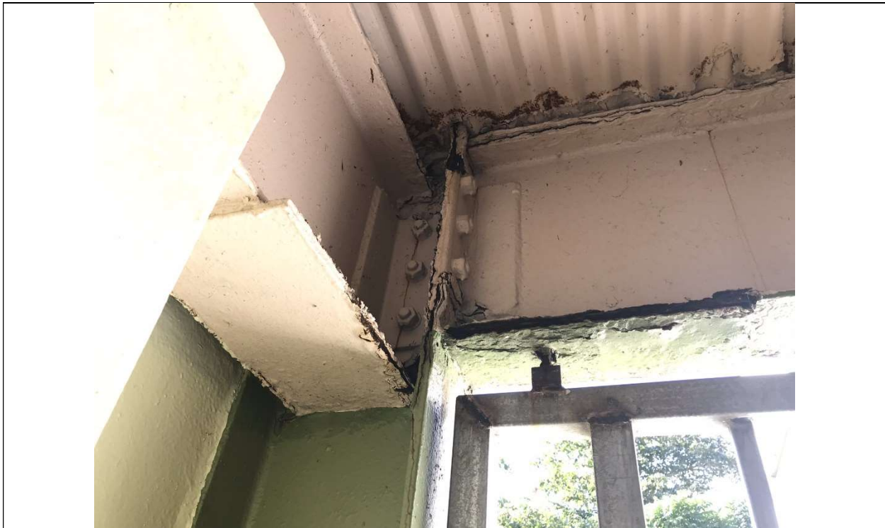
Picture 8 - Steel structure connections and sections with advanced corrosion conditions
