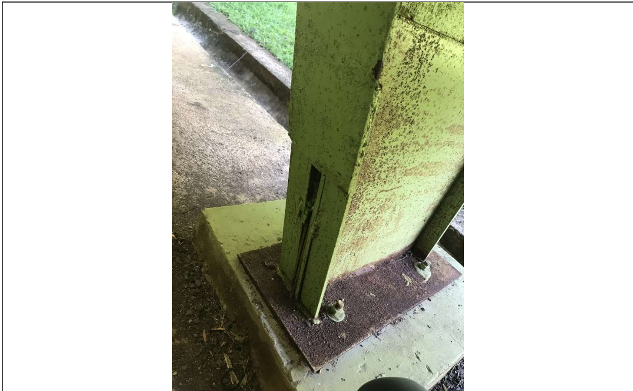
Picture 14 - Basketball Court - All main steel columns (4ea) of the West exterior axis were previously repaired by: (1) Cutting approx. 6" to 24" of the column bottom and replacing it with a questionable detail using angles and plates with various welding segments and (2) Replacing the base plate with a thinner plate and new smaller diameter anchor bolts.
