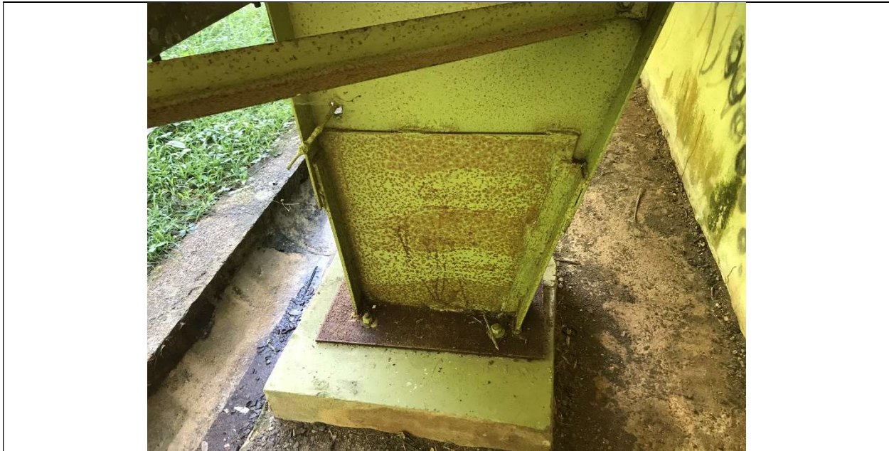
Picture 13 – Basketball Court - All main steel columns (4ea) of the West exterior axis were previously repaired by: (1) Cutting approx. 6" to 24" of the column bottom and replacing it with a questionable detail using angles and plates with various welding segments and (2) Replacing the base plate with a thinner plate and new smaller diameter anchor bolts.
