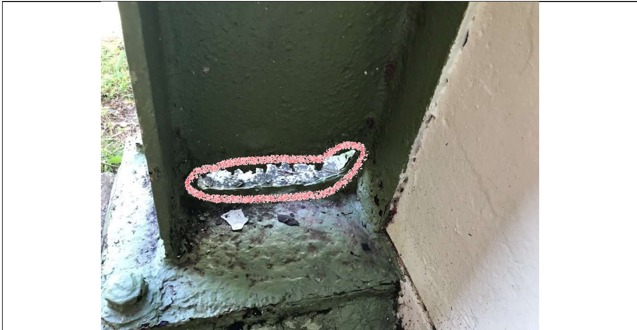
Picture 3 – Steel columns significant loss of metal at web and flanges within 12" of the plate due to extreme corrosion - Exterior perimeter columns
