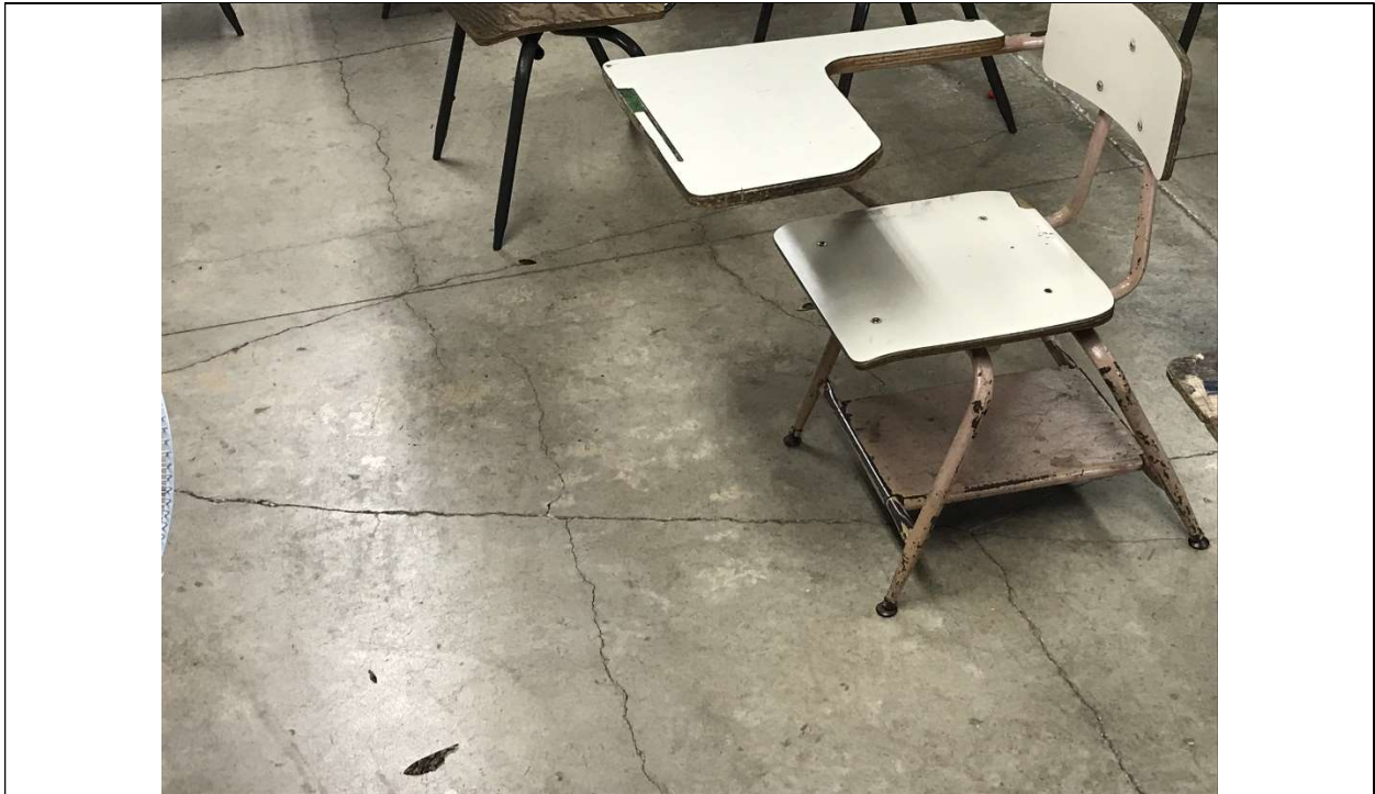
Picture 15 - Slab cracks random patterns in many of the classrooms (all levels)
