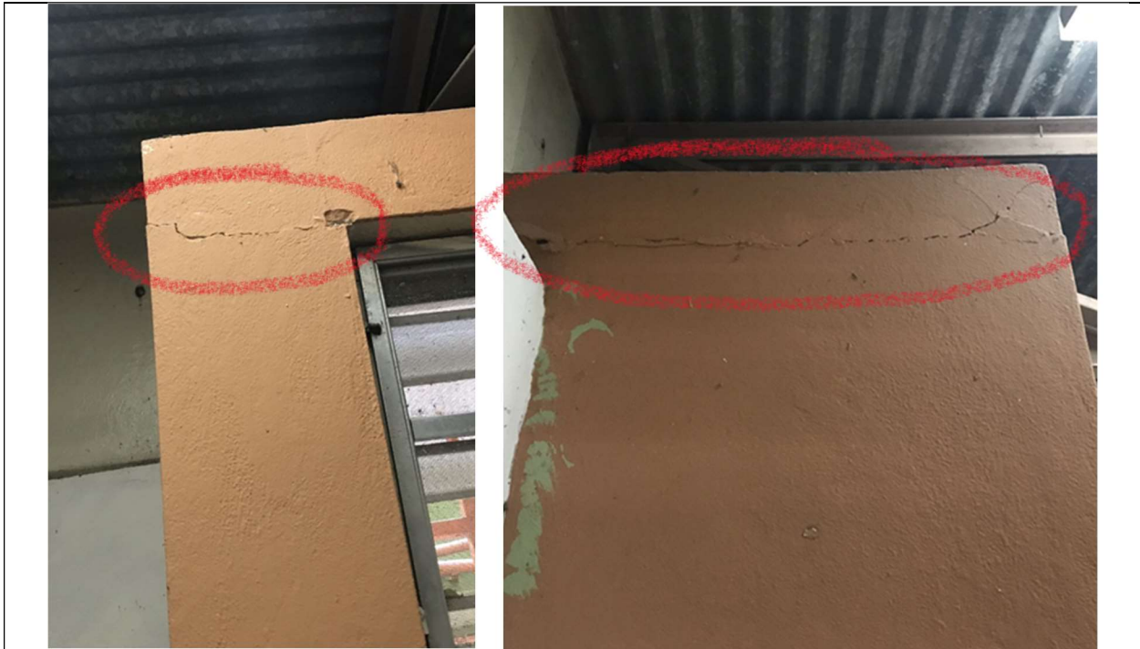
Picture 12 - Horizontal crack on left side of the vertical-horizontal connection of a windows concrete casing in the dining hall area
