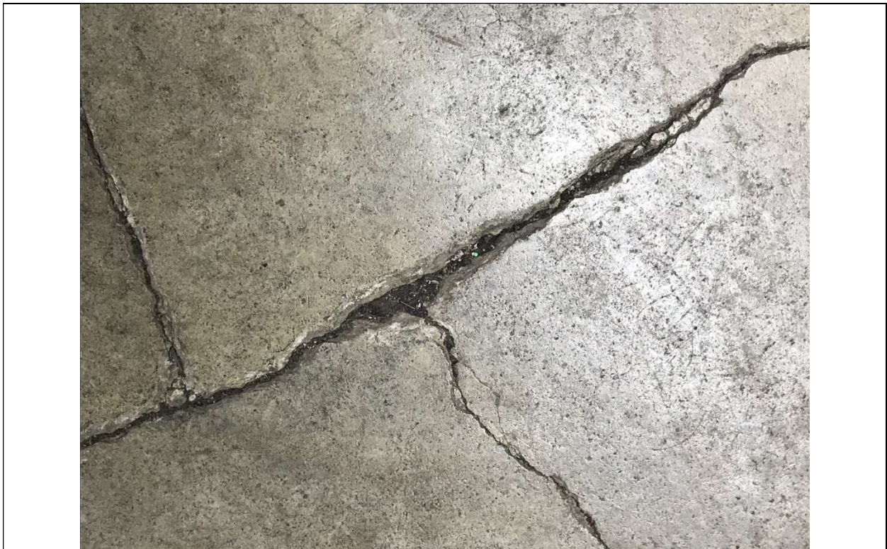
Picture 16 - Slab cracks random patterns in many of the classrooms (all levels)
